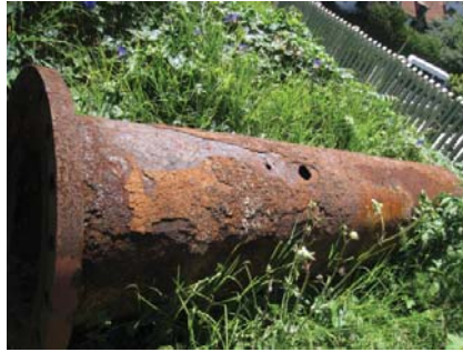
TOP Delamination and corrosion of the existing steel pipe
