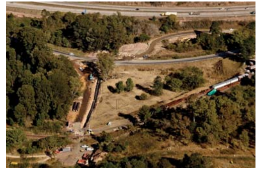
An aerial image showing the progress of construction in the vicinity of Inchanga Station – part of Phase One of the Western Aqueduct Project, which is almost 80% complete
