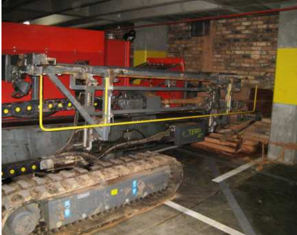
The Terra Jet 7520 with the automatic drill-loader removed, drilling in the confined basement
