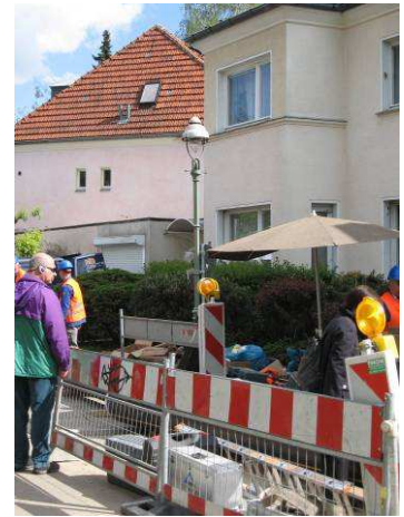
A real gas-fuelled street lamp in the 21 st century!
