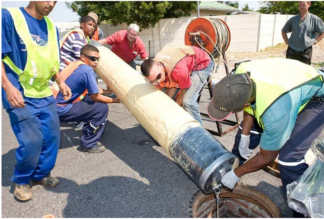
The liner has been wrapped onto the bladder, which will shortly be inserted down the manhole and into the sewer pipe.
